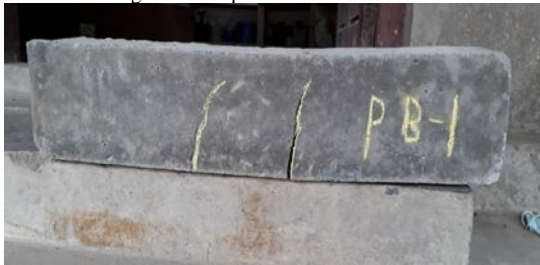
Fig. 10. Crack pattern of PB 1
