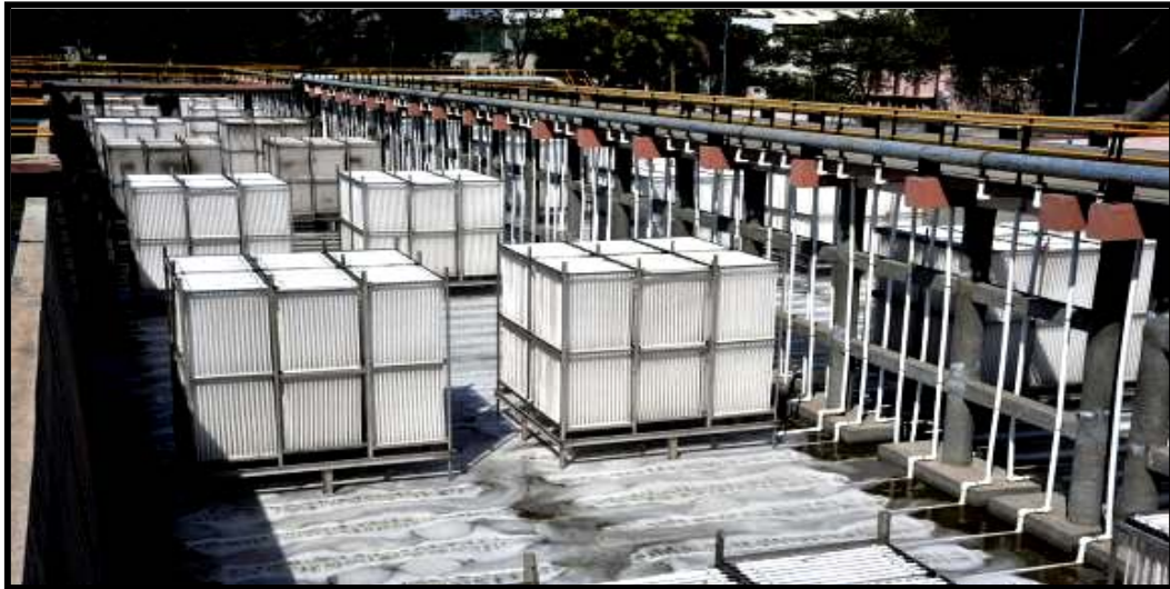
Fig. 4 Equalisation tank of 100 MLD STP, Bamroli modified to IFAS system
