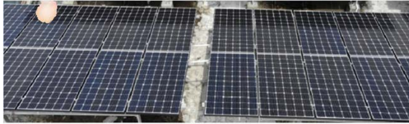
Fig. 9 Failures of solar panel map
